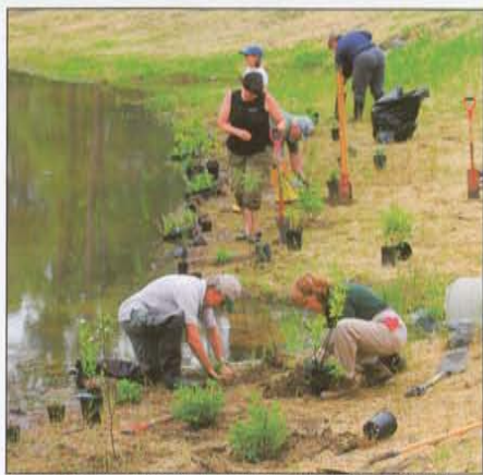
Volunteers install a wetland buffer around the edges of a stormwater retention pond at Union Bank Shares in Caroline County.
