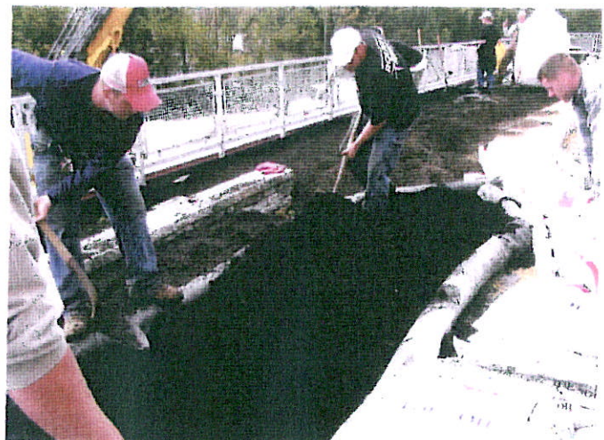
Planting areas with 3- to 9-inch depths were installed on the green roof depending on intended type of vegetation.
