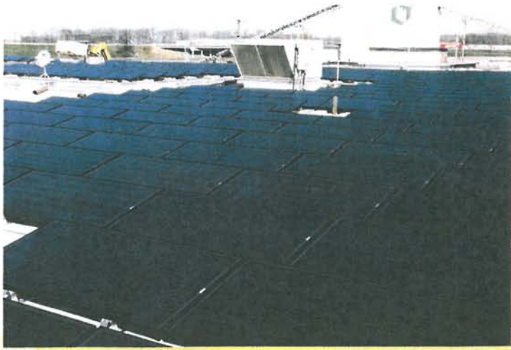
A total of 572 solar panels installed on the WSSI roof supply nearly 21 percent of the facility's monthly energy supply.
