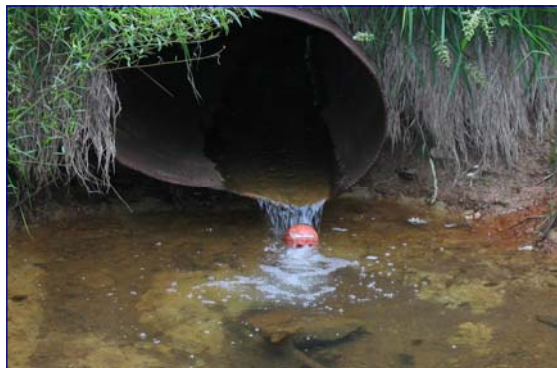
SEVERE - Piped (culverted stream)
