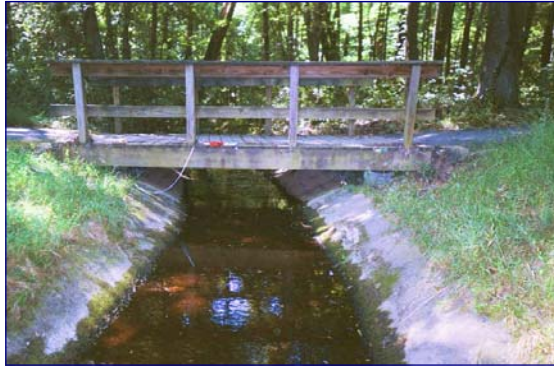
SEVERE - Concrete lined channel causing permanent disturbance to Waters of the U.S.
