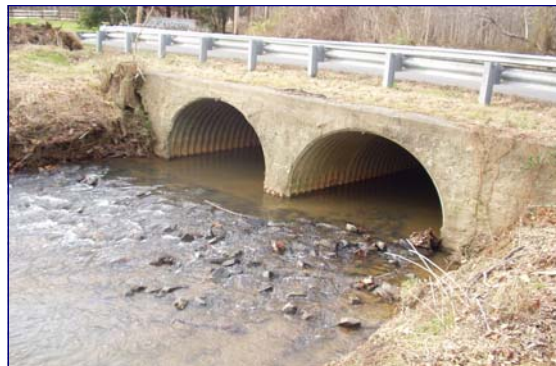
SEVERE - Twin-CMP Arch culverts with concrete bottom
