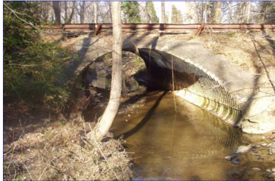
SIGNIFICANT - Countersunk culvert
