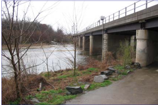
MODERATE - Bridge with multiple piers causing permanent impacts to Waters of the U.S.
