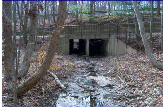
SEVERE - Box culvert impacting stream bed
