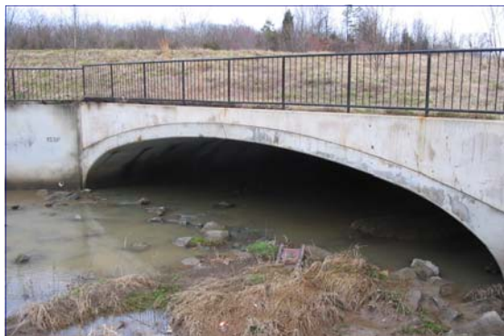
SEVERE - Bottomless culvert with scour protection
