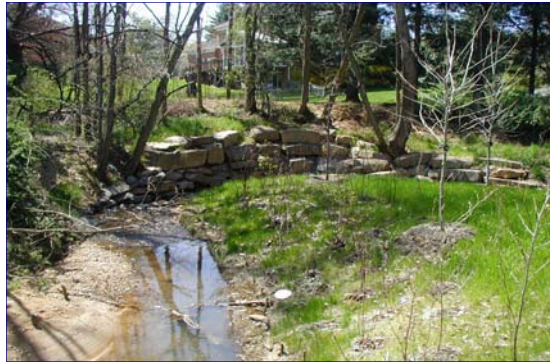
RF = 2.25: Northern Virginia, Urban/suburban stream utilizing bio-engineering techniques on one bank. The right bank was regraded with biologs placed at the toe of the slope and the bank was replanted with native vegetation. Left bank has one segment of imbricated stone to save trees.
