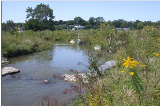
RF = 3.50: Western Maryland, Rural stream restored utilizing Natural Channel Design techniques and grade control structures.
