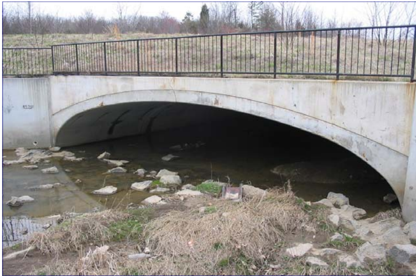
IMPACTS 3, 4, 5 - Bottomless culverts with scour protection.
