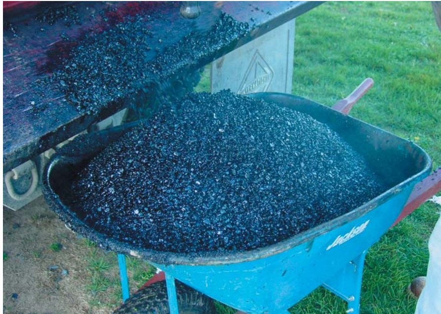
Fig. 1.27 Porous Asphalt straight off the truck for installation at the Cornell Test Plots. Note the absence of fine particles within the asphalt mix.
