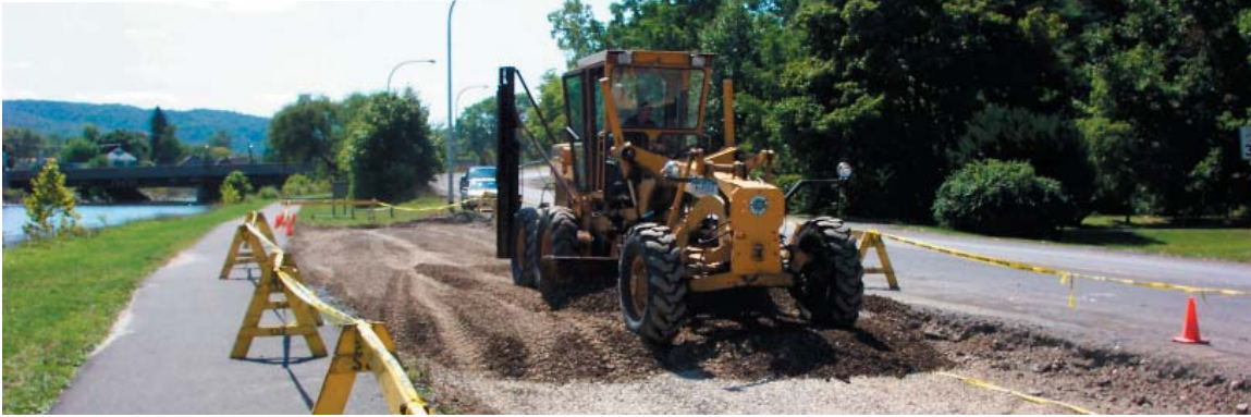
Fig.1.12 Grading of CU-Structural Soil® used as the reservoir base course for porous asphalt lot in Ithaca, NY. For this lot, 2' of CU-Structural Soil® was used to hold a 100 year storm event of 6" in 24 hours.
