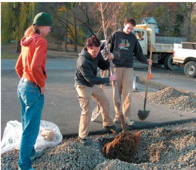
Fig. 1.25 Students planting bare root Ulmus japonica x Ulmus wilsoniana 'Accolade' (Accolade Elm) in the apron containing CU-Structural Soil® surrounding the porous asphalt parking lot in Ithaca, NY in November 2005.
