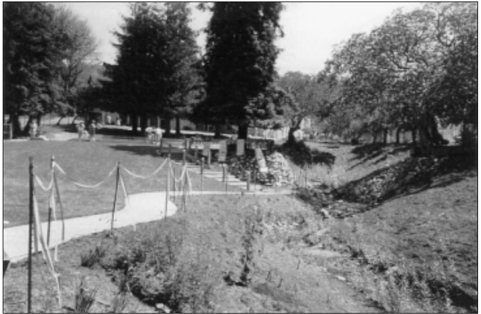
The Blackberry Creek site as it appeared in 1996. Crews daylighted and planted the site in late 1995. Courtesy of Wolfe Mason Associates.
