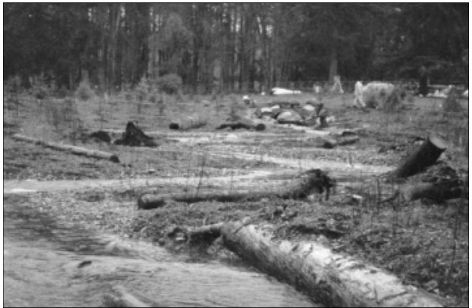
A section of Jenkins Creek shortly after daylighting, showing meanders and newly installed habitat features such as root wads and control logs. Courtesy of Ken Nilsen.
