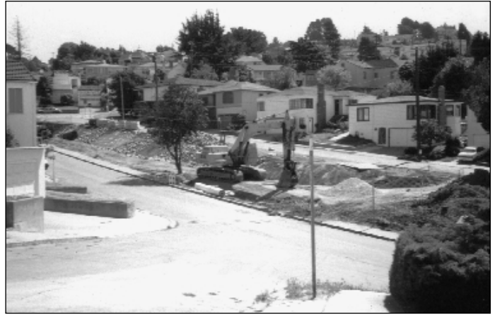
Construction of the Baxter Creek daylighting project at a hillside park in El Cerrito, California in 1996. Courtesy of Lisa Owens-Viani.
