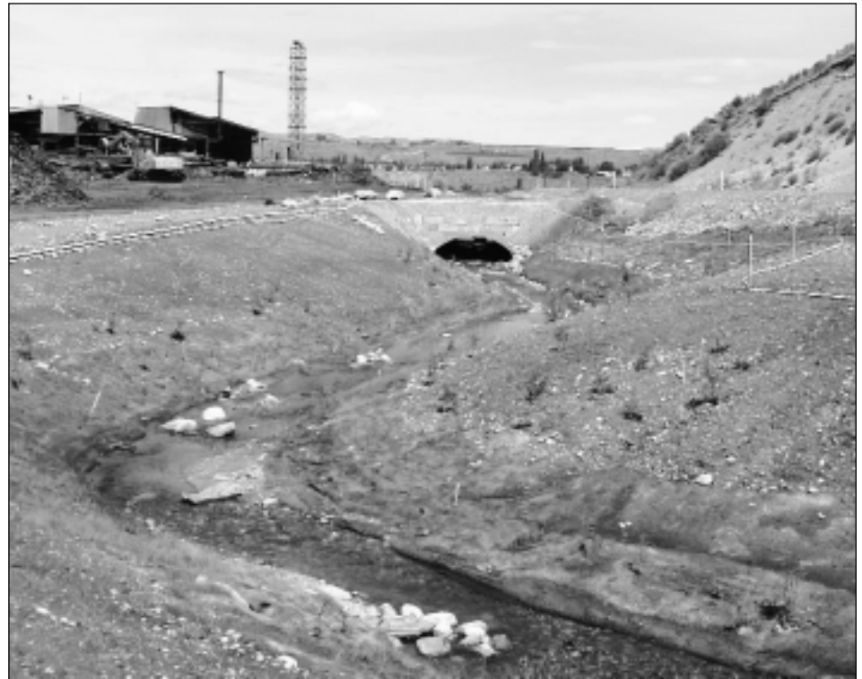
A portion of the daylighting project by the Quality Veneer & Lumber mill in Omak, Washington, a few months after completion in 1999. Vegetation is just beginning to take hold. The new “bottomless culvert” in the upper middle of the photo spans a short stretch of the opened stream. Courtesy of Ridolfi Engineers.
