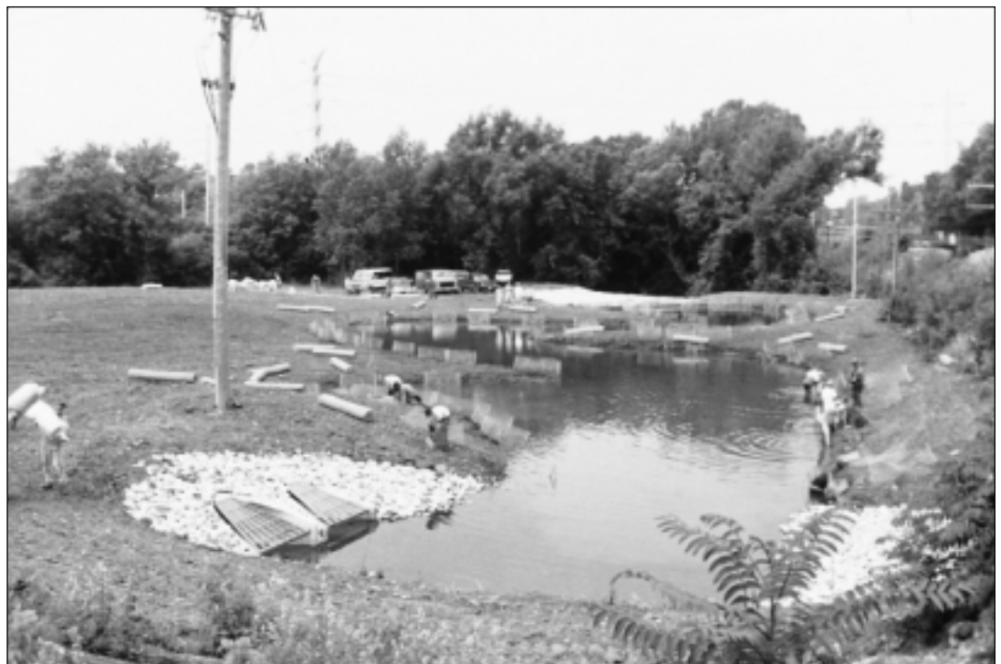
Kilgoblin Wetland after construction. Crews seed the banks, install protective cages around plantings, and prepare to roll out erosion control blankets. Grates cover the two culvert outfalls in the lower left. Courtesy of Village of Barrington Department of Public Works.
