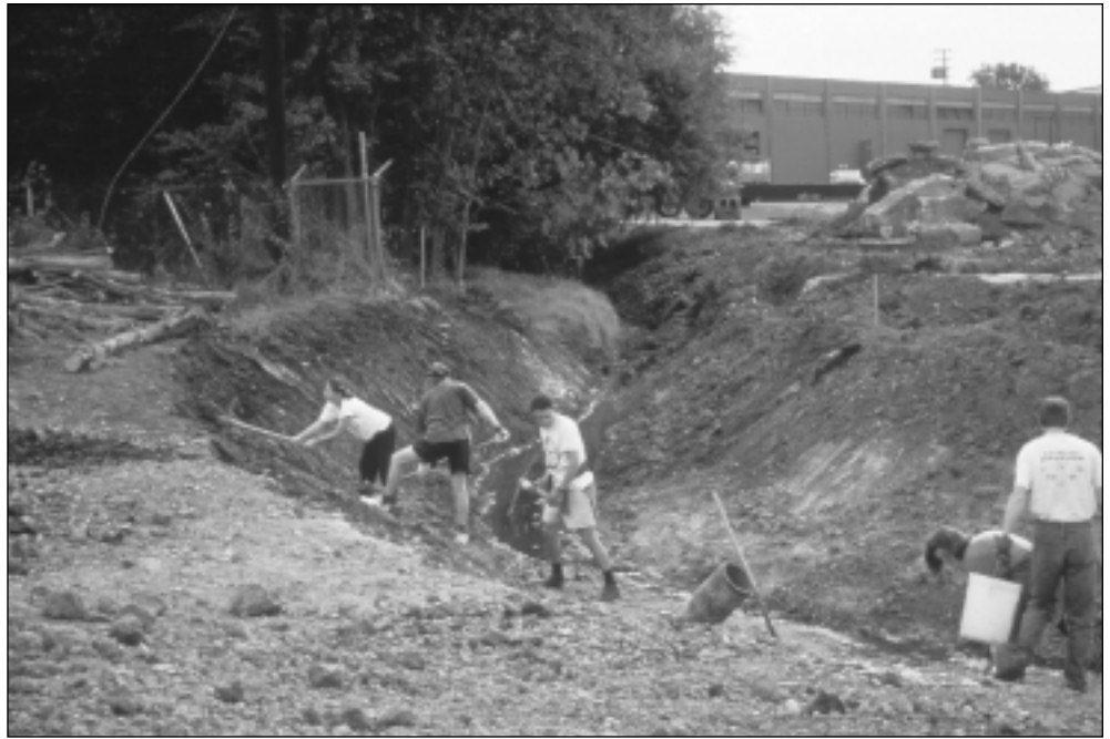
Volunteers working on the banks of the new Codornices Creek channel shortly after excavation. Courtesy of Wolfe Mason Associates.
