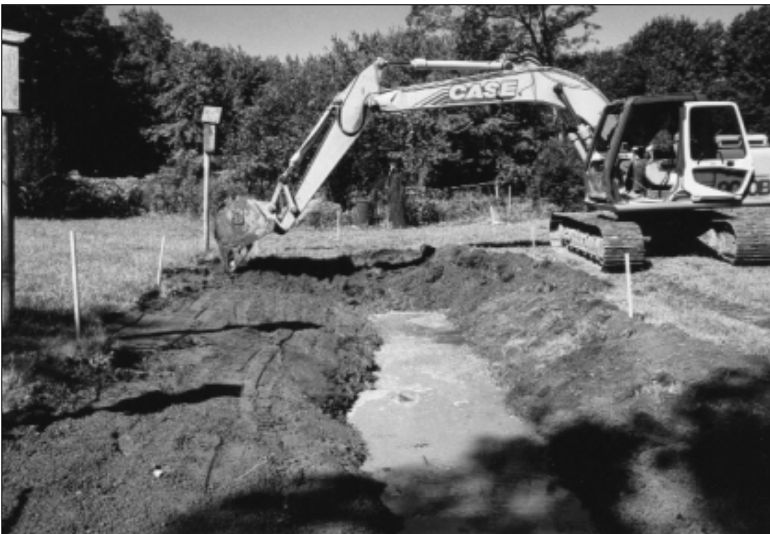
A backhoe halfway through removing a culvert and grading the banks of West Ox Pasture Brook in a Rowley, Massachusetts backyard. Courtesy of Rowley Conservation Commission.
