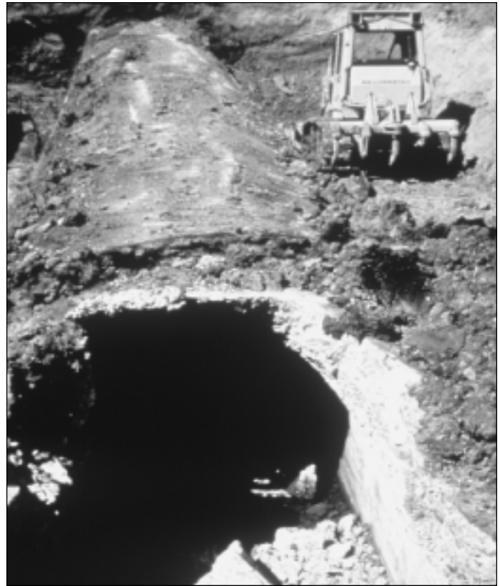
Removal of the culvert at Strawberry Creek in Berkeley, California in 1984. Courtesy of Wolfe Mason Associates.
