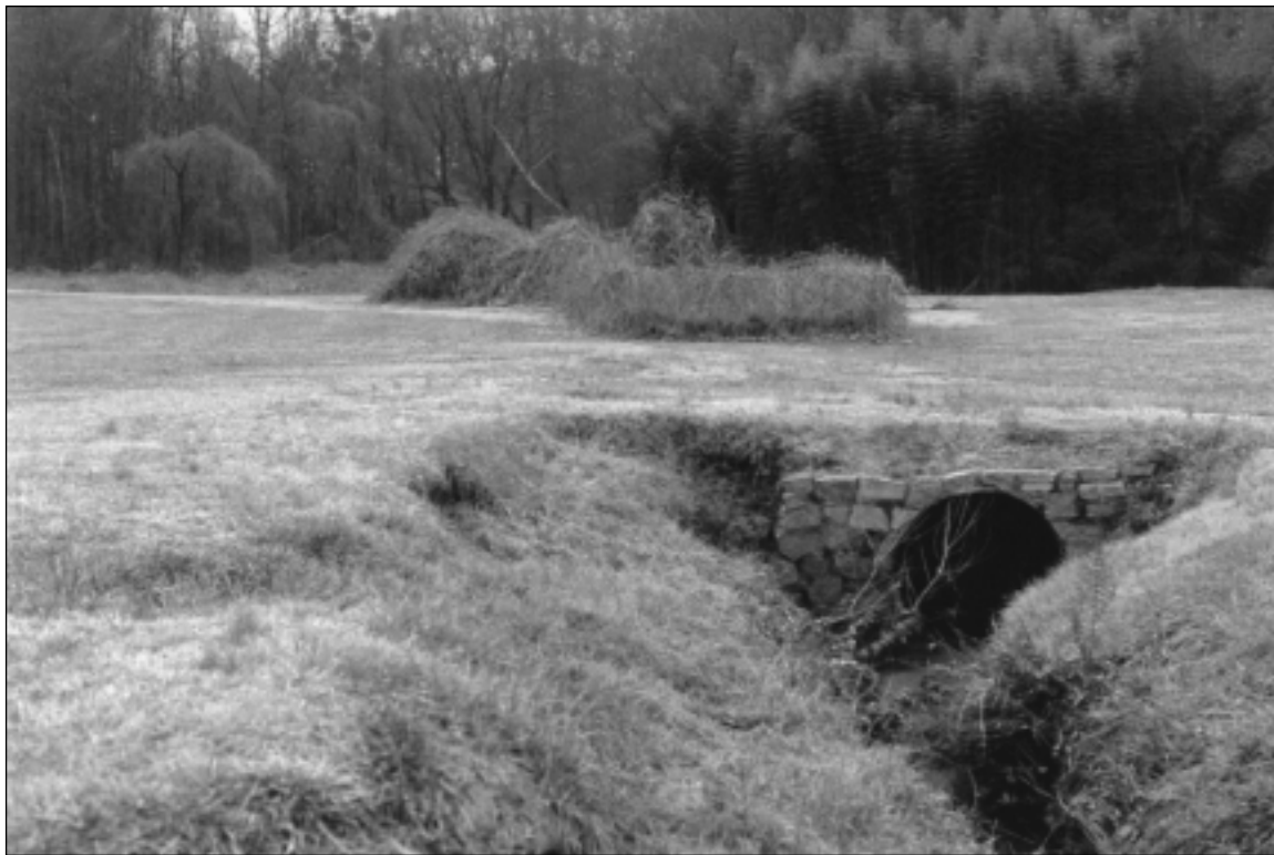
A culverted creek in Longdale Park near Atlanta prior to daylighting. Kudzu vines crawl over fences around collapsed sections of culvert. Courtesy of DeKalb County Parks Department.
