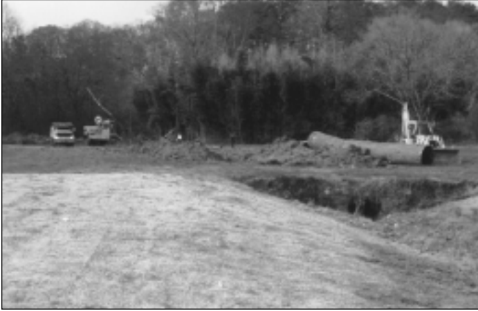
Daylighting is often a good, low-cost solution for collapsed culverts. This 1994 project near Atlanta, Georgia replaced a deteriorating metal pipe with an open, naturalized channel. Courtesy of DeKalb County Parks Department.
