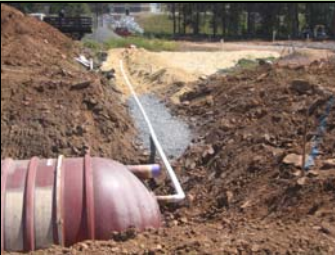
Rain garden pipes, Sept. 2005
