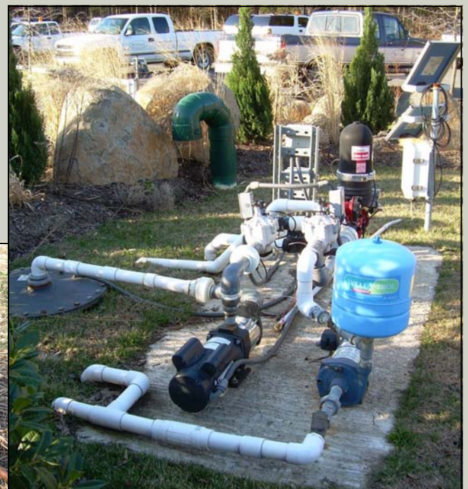
Irrigation equipment and cistern vent
